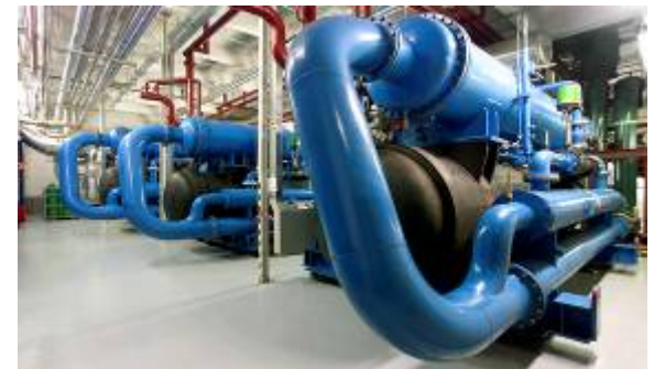
30 MW cooling capacity
